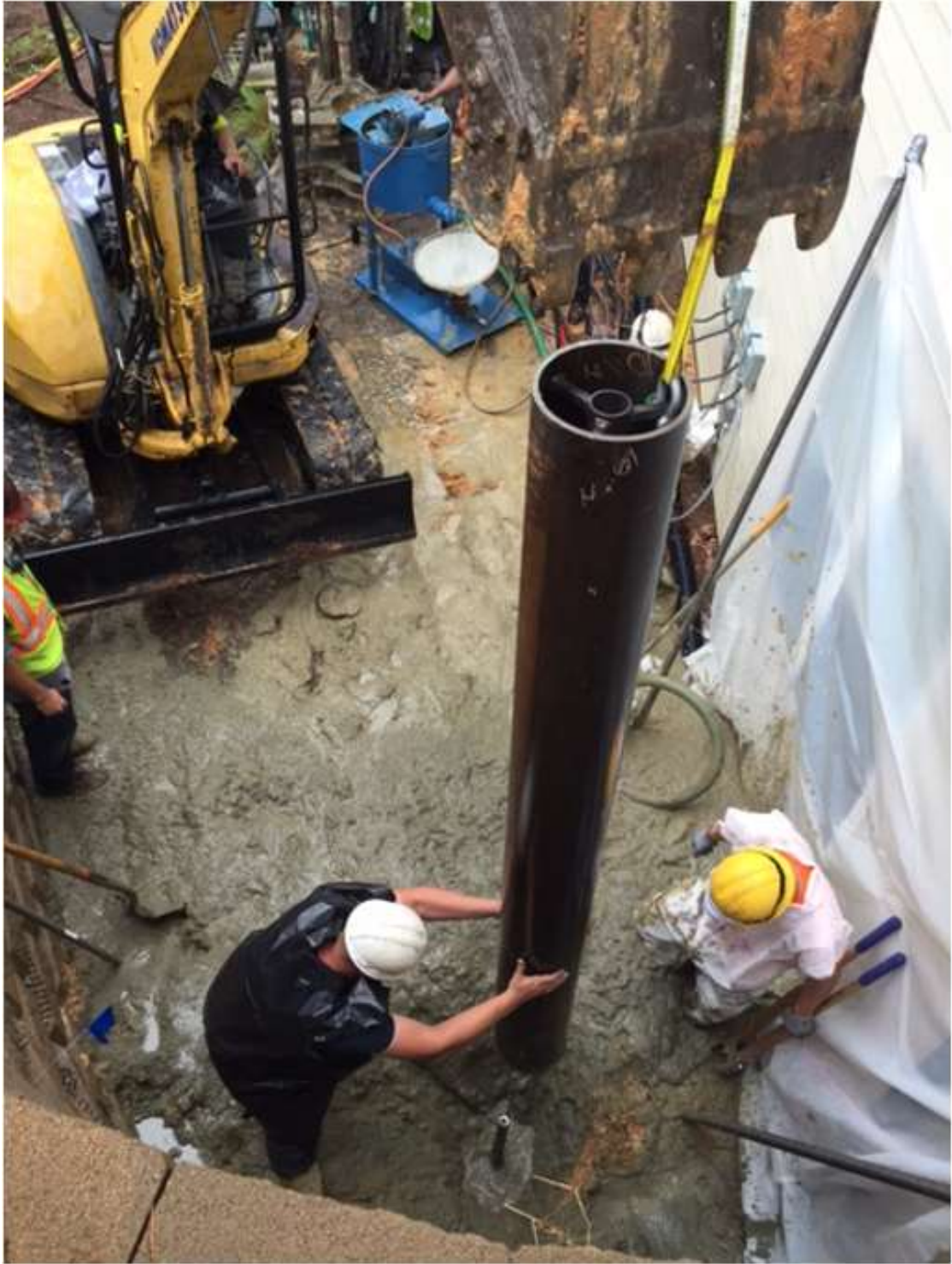
Figure 4. A cased section is lowered into the drilled and grouted hole. The casing is aligned along the center bar with a series of collars within the casing.
