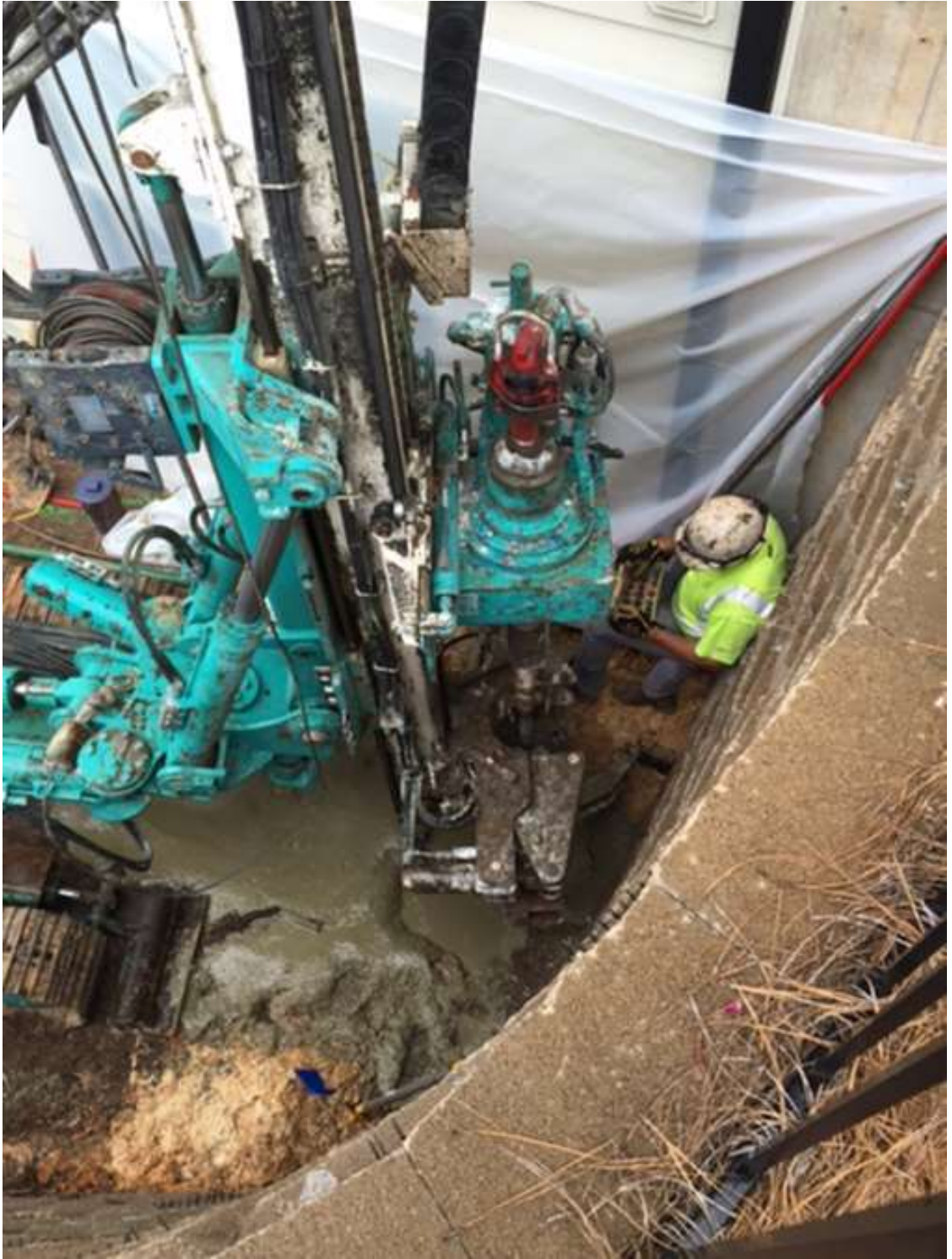
Figure 1. Viewing down from the top of the adjacent retaining wall, the installation of one of the micro-piles can be seen.
