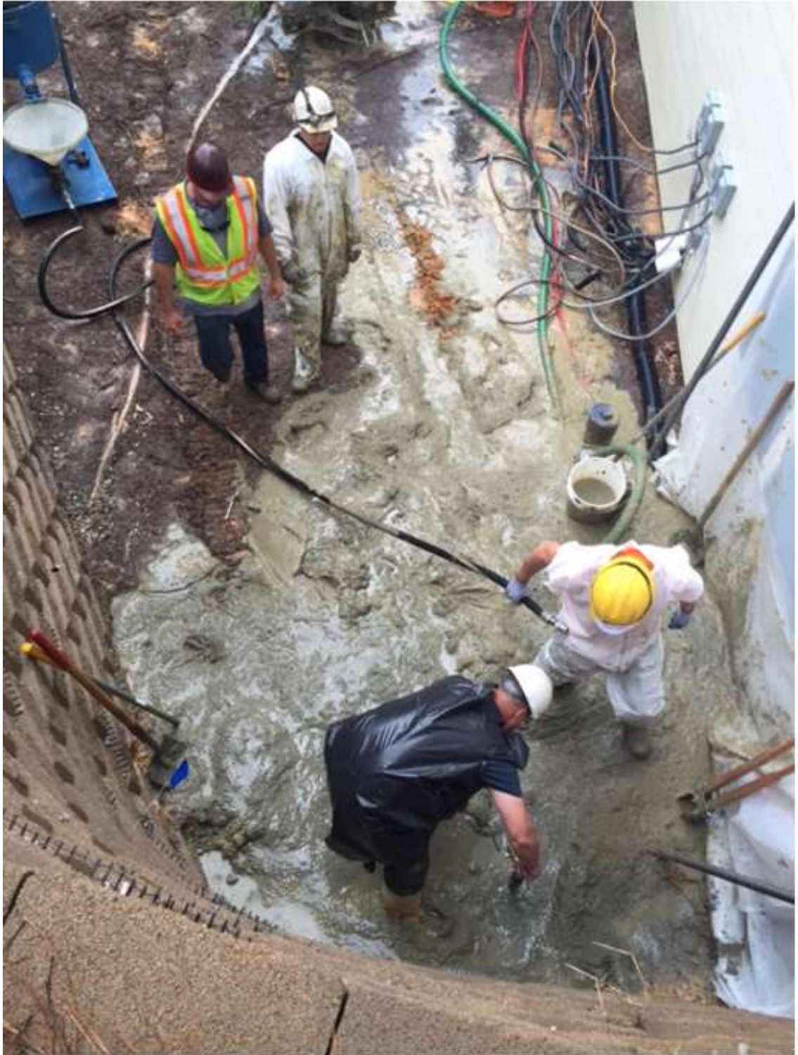
Figure 2. After drilling, the grout is pumped from the center of the bar.
